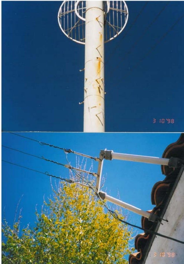
Figure 16: Monopole and Slant Wire Lower Termination at Triplexed Antenna in Santa Barbara, CA.
