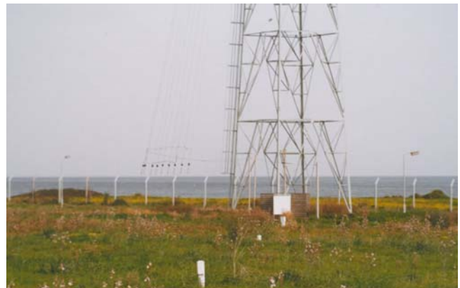
Figure 24: Slant Wire Feed and ACU Enclosure
